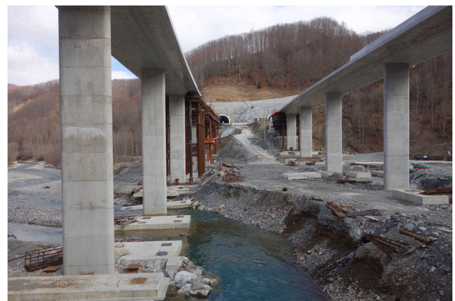
Fig. 4. Construction site at the river Tara. Photo taken by the first author on road R-13 near Mateševo on February 22, 2020.
