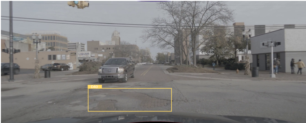
Figure A.5: Pothole (D40) in an example image of the ADS (USA)
