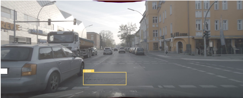
Figure A.1: Aligator crack (D20) in an example image of the ADS (Germany)
