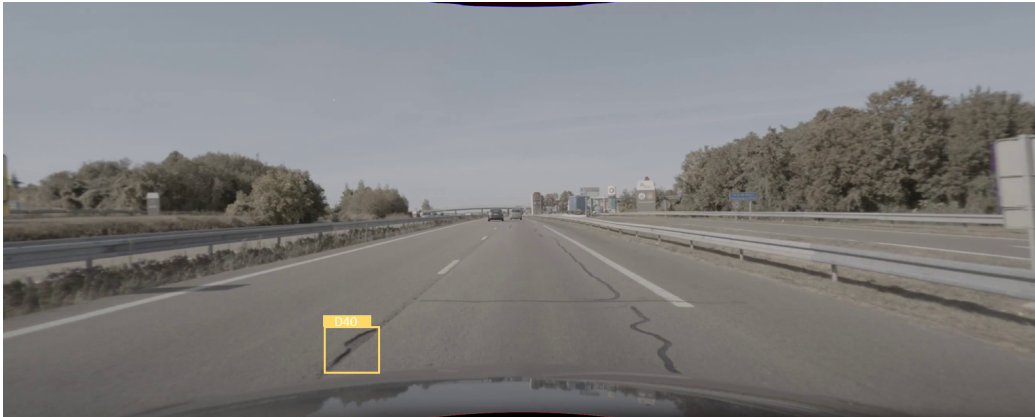
Figure A.7: Pothole (D00) in an example image of the ADS (France)
