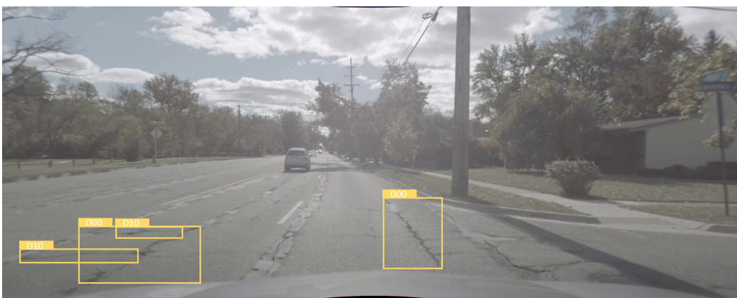
Figure A.3: Multiple damages in an example image of the ADS (USA)
