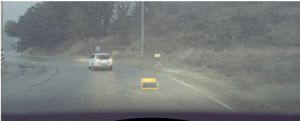
Figure A.11: Pothole (D40) in an example image of the ADS (South Korea)
