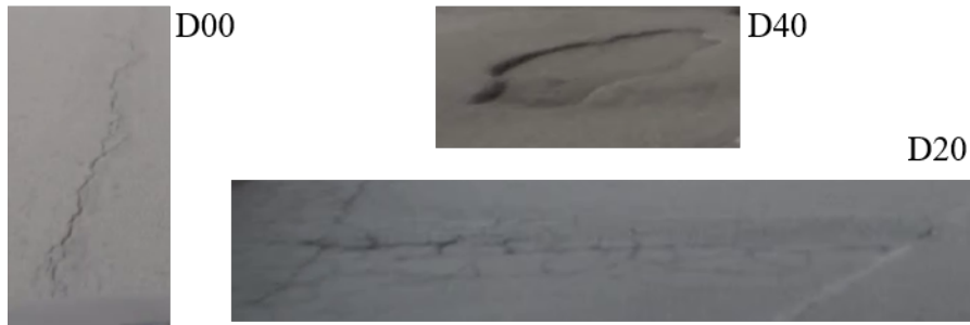
Figure 2.10: Road damages drawn from the example images in Appendix A
