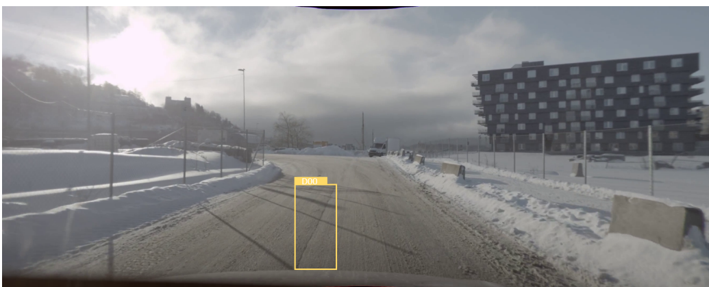
Figure A.9: Long. crack (D00) in an example image of the ADS (Norway)
