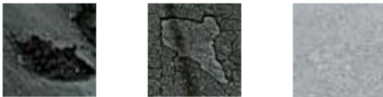
Figure I.7: Examples of high, medium and low severity potholes
