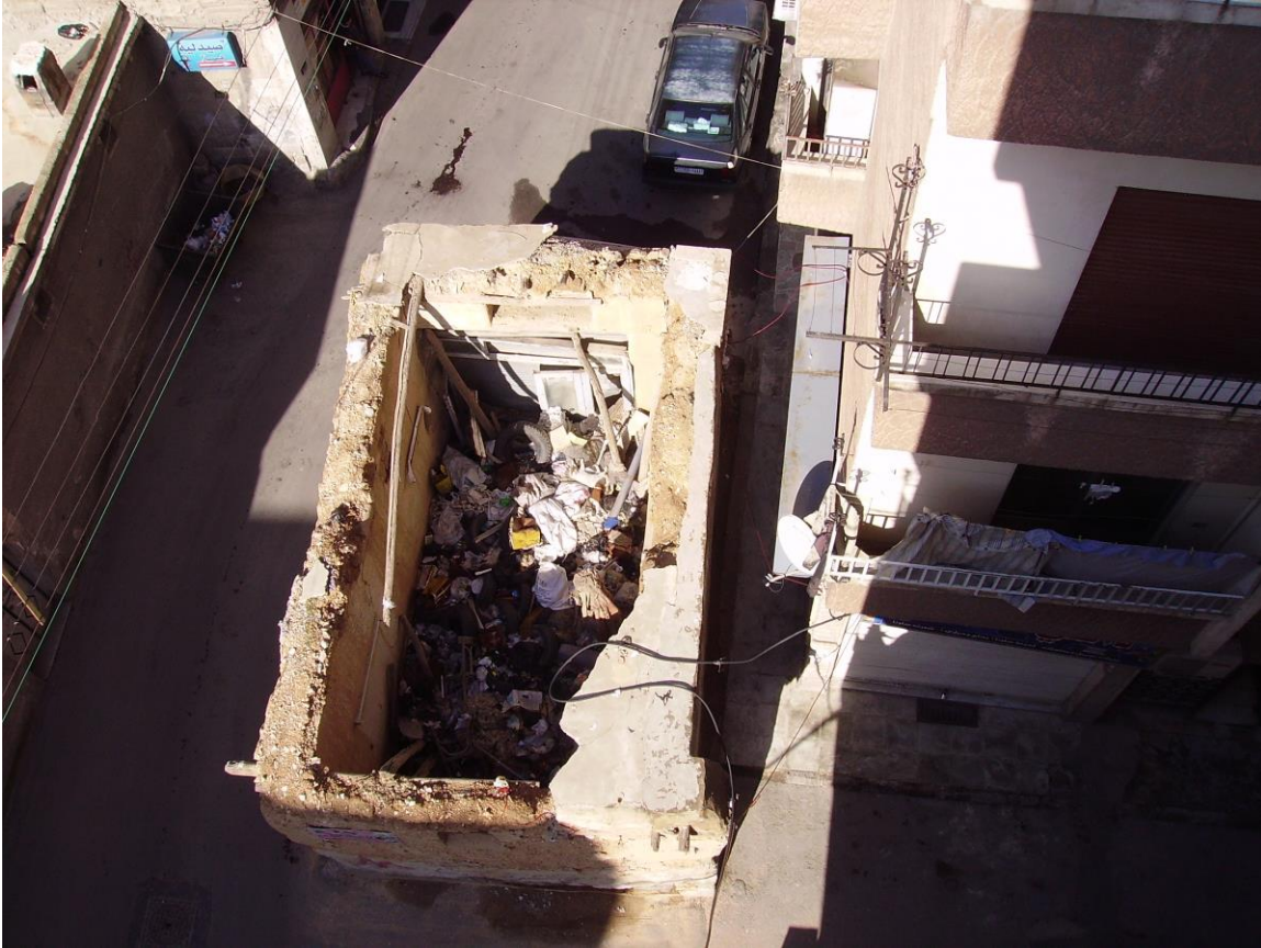
Having no roof, the abandoned store became a source of health hazard. (2010, by the author)
