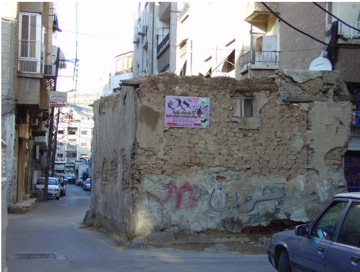
Site 722 blocking a large section of the street, causing different forms of harm (2010, by the author)
